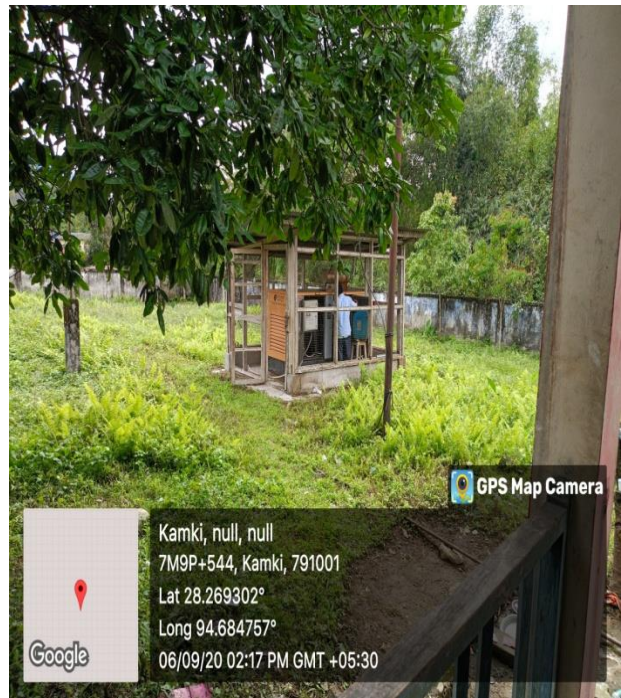
(Diesel Generator Set)
